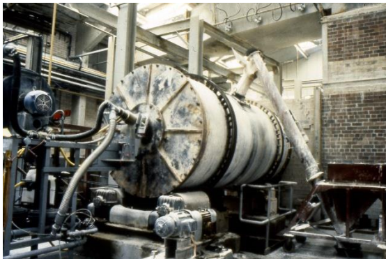
Furnace being charged from ground level hopper through screw conveyor,
