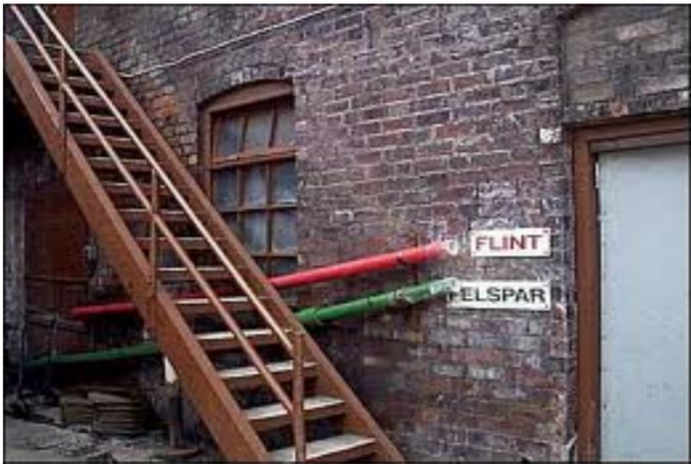
At the customer end, suitable pipework may be provided, as can be seen as example in the photograph, left.
